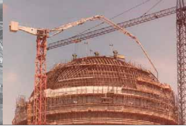
Trillo I Nuclear Power Plant
