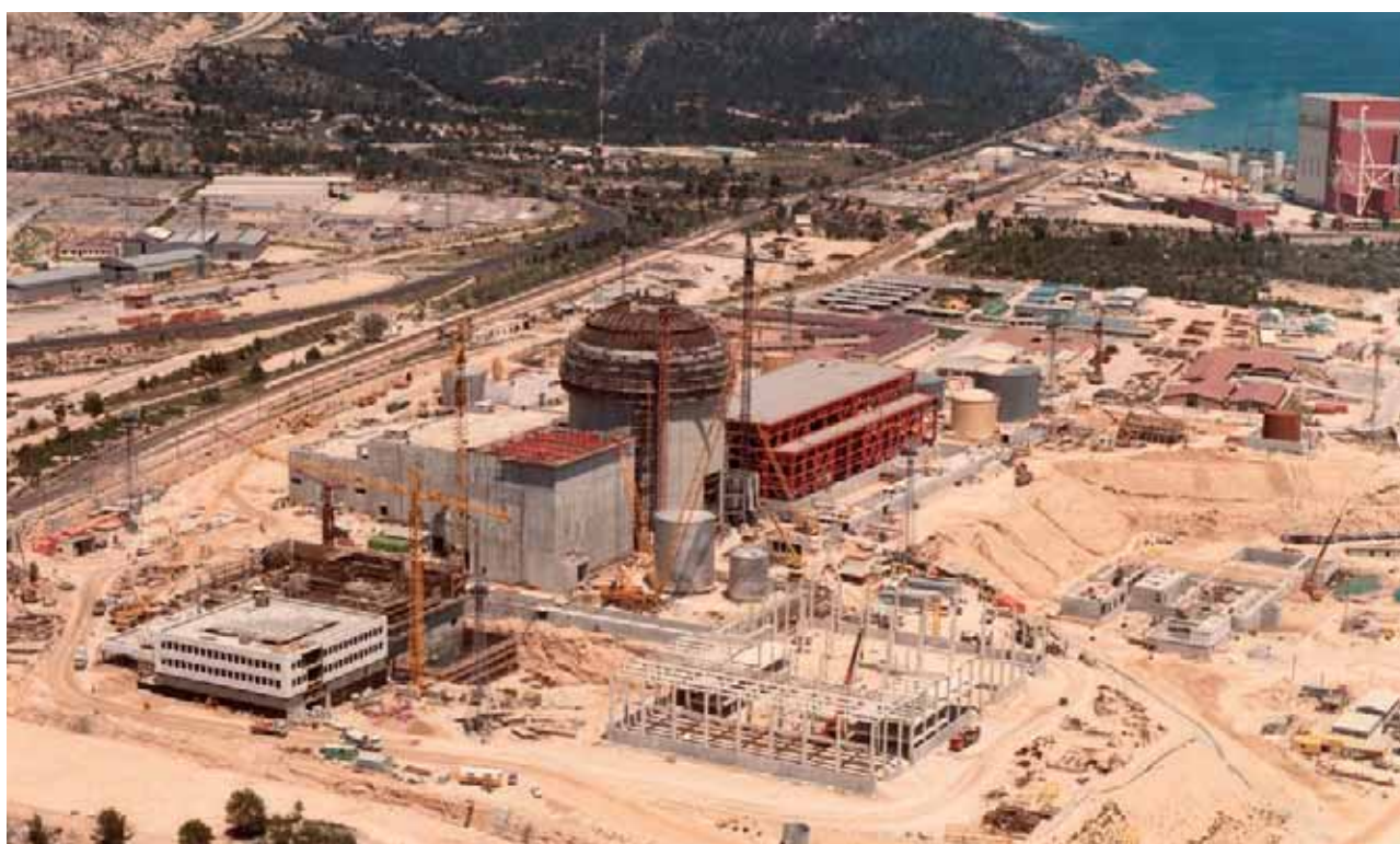
Construction of Vandellòs II Nuclear Power Plant with Vandellòs I in the background
