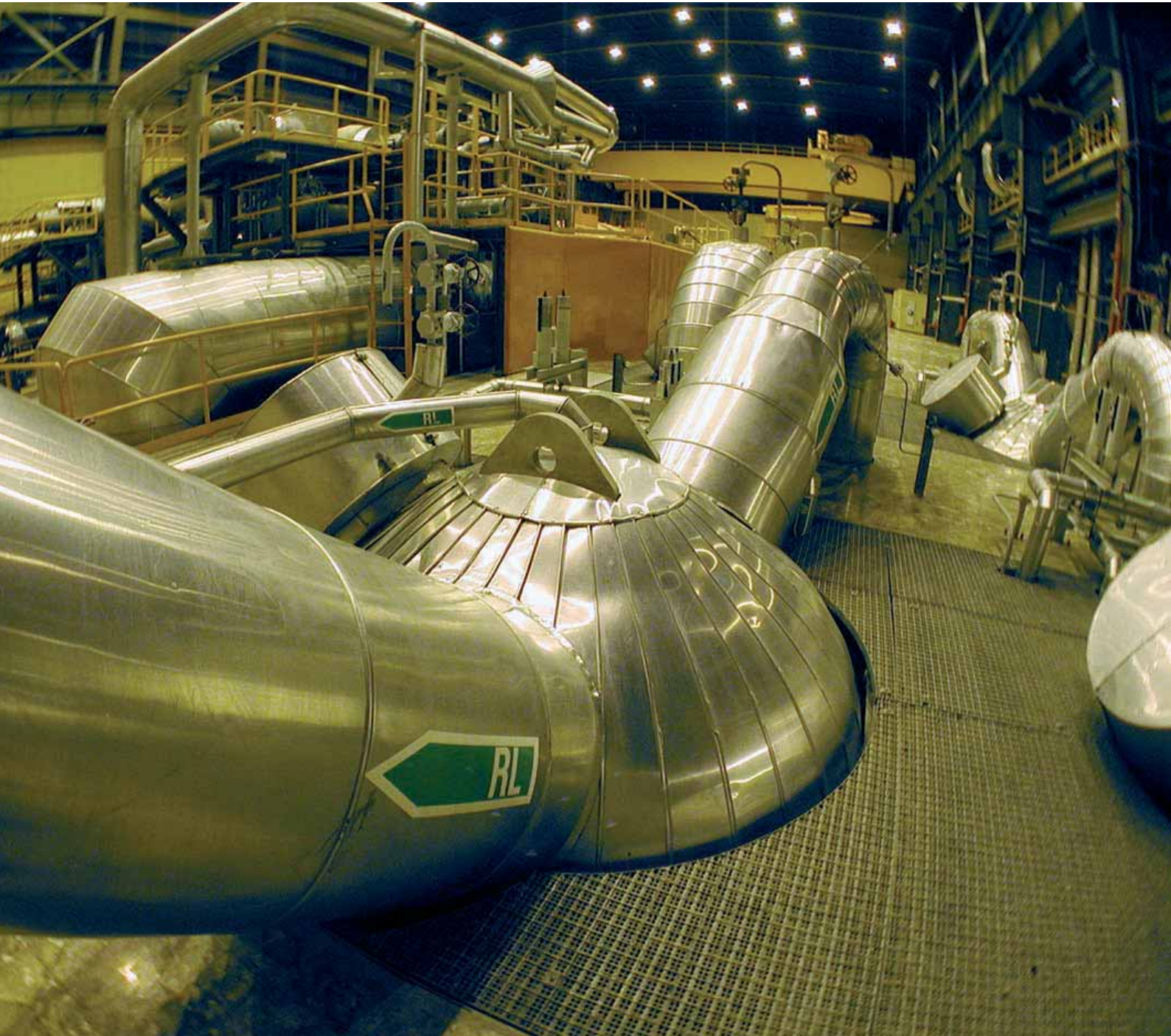
Turbine Building of a Nuclear Power Plant
